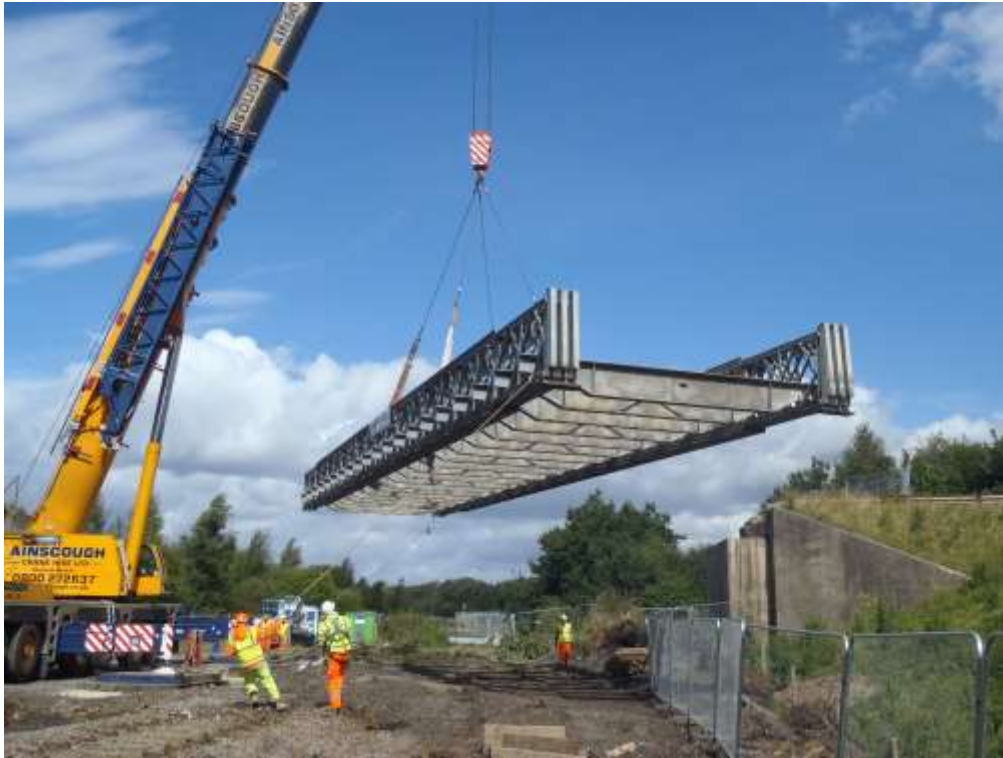
Demolition of a redundant 'bailey bridge' over Erin Road and the disused Bolsover branch line
