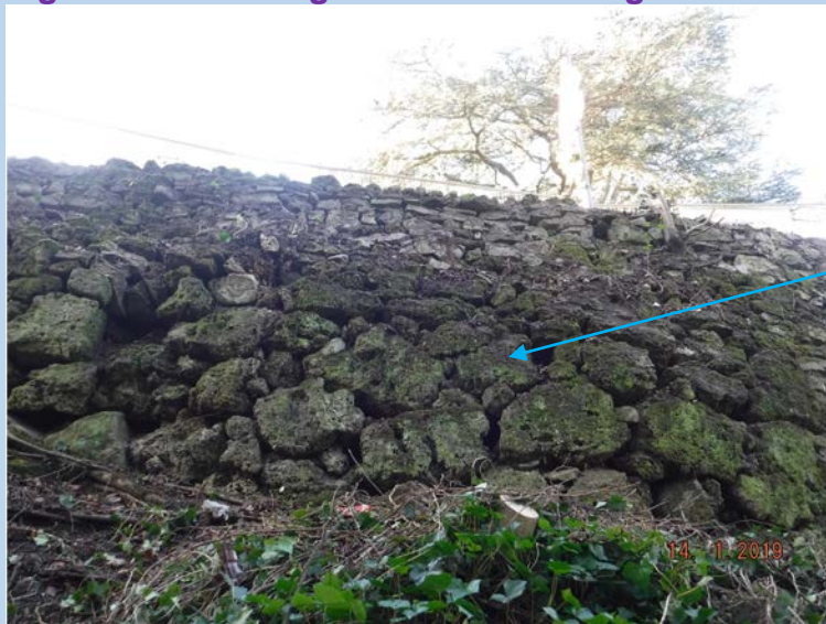
Figure 1 – Showing Failure of Existing Structure
