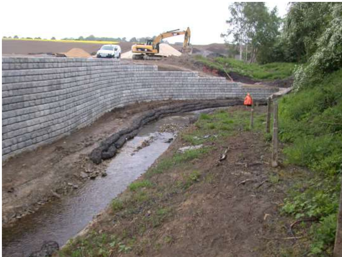
Diversion of the Hawke Brook and construction of a retaining wall to create development plot above.
