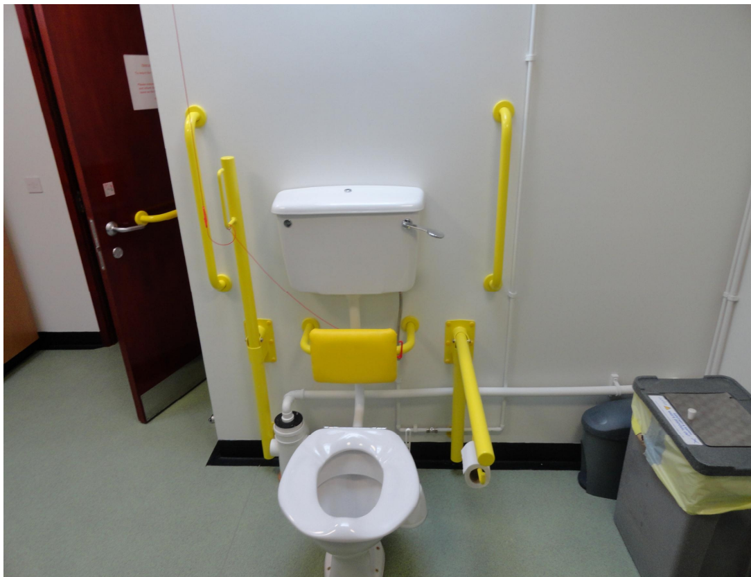
WC and colour contrasting grab rails
