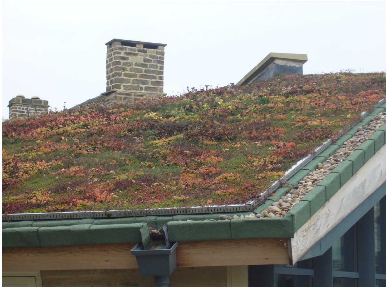
Green roof planted with sedum and drought tolerant species
