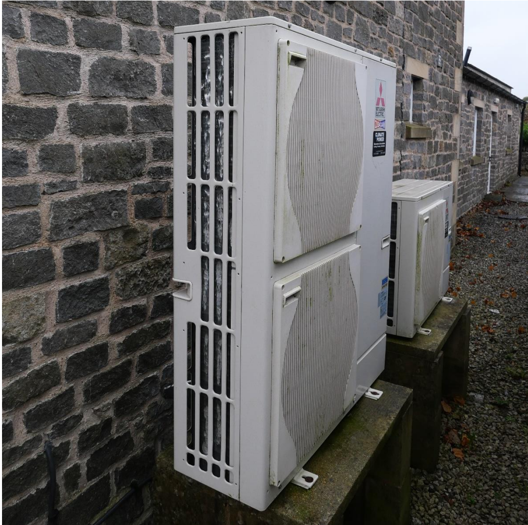
Air source heat pumps, Over Haddon Village Hall, Derbyshire. Image with permission of Over Haddon Village Hall.
