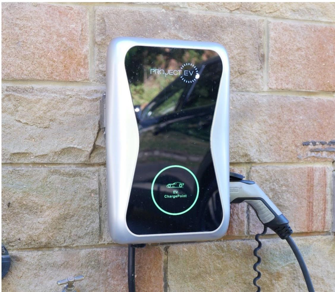
7.3 kW domestic electric vehicle charge point.
