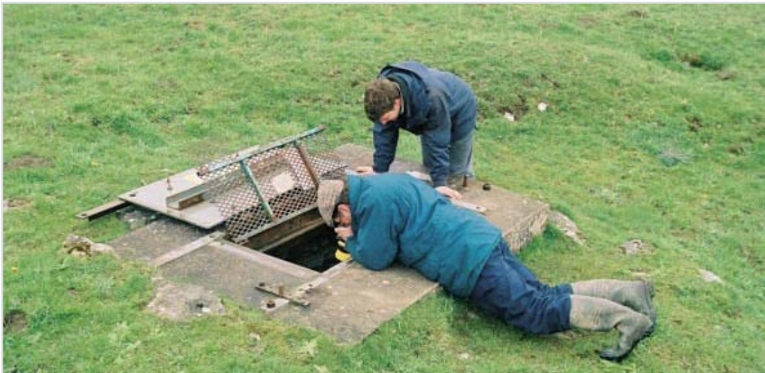
A secure hinged grille can provide access to a shaft
