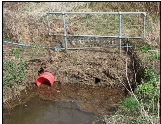
A blocked culvert
